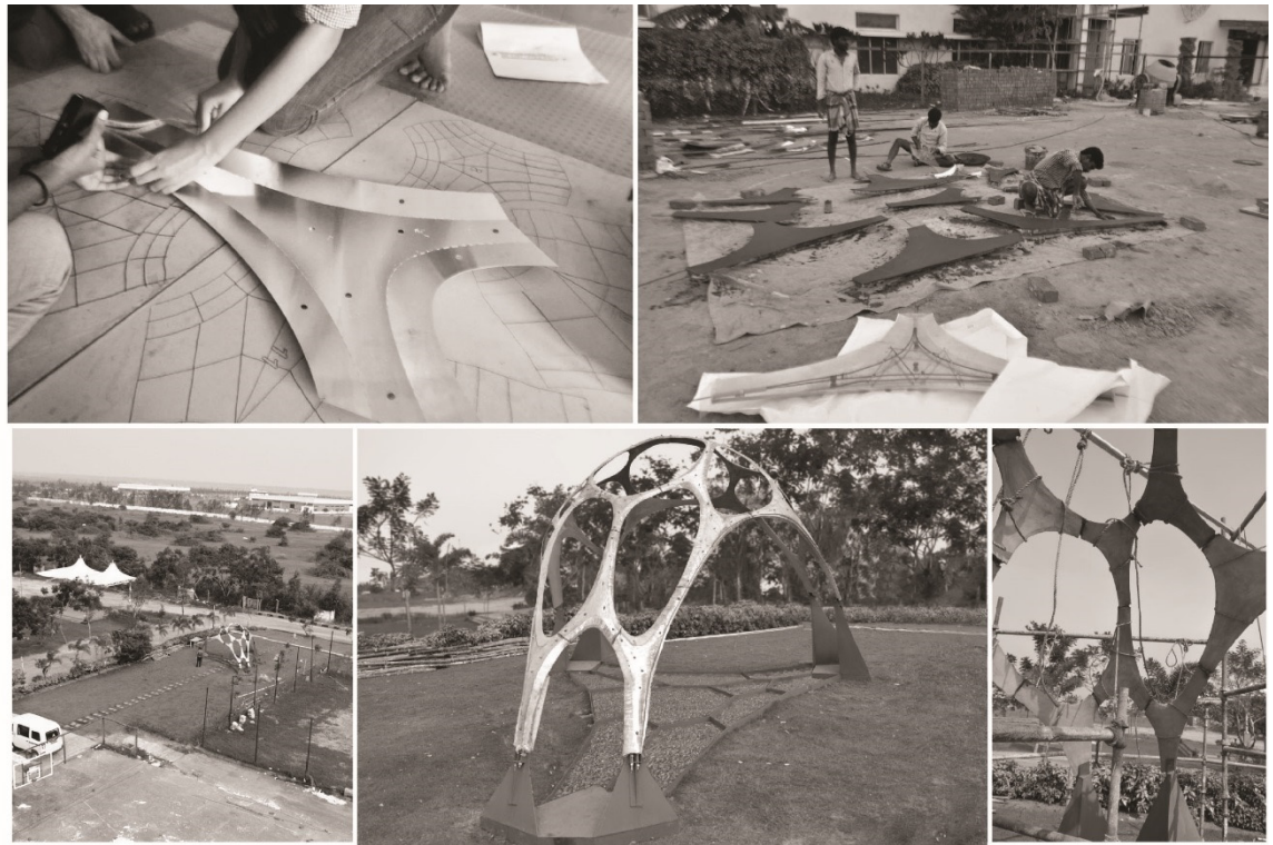
Figure 57 Construction of a funicular skeleton structure using CCF moulds. Image courtesy (S Bhooshan, Bhooshan, et al. 2015)
