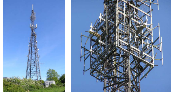
Figure 2 Bathampton DAB and DVB-T transmitter near Bath. Left: transmitter tower. Right: close-up of array.
