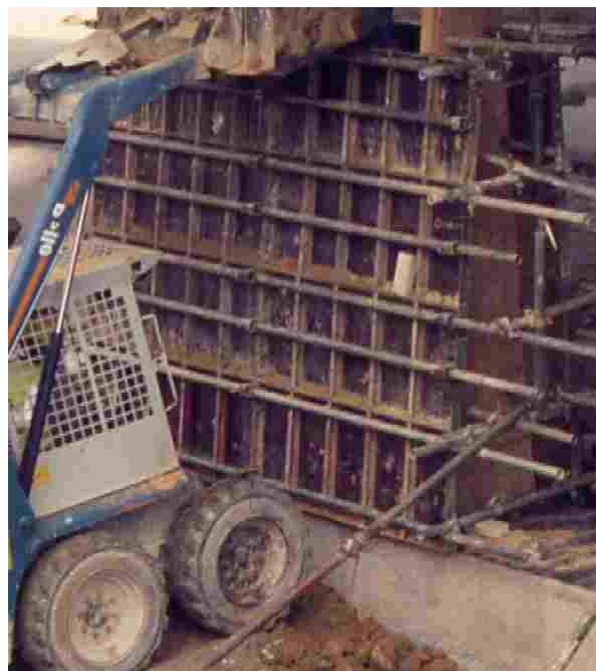
Figure 6.3: Battered formwork at Eden Project (photo: R. Keable)
