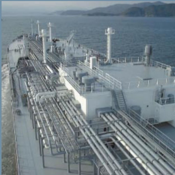
LPG (Liquid Petroleum Gas) 'MV Anne Laure' fitted with complete Hamworthy KSE cargo handling package: reliquefaction plant, deepwell pumps and inert gas generator system.
